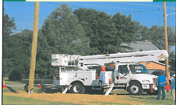
New Electrical Service—North
