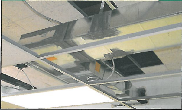
Duct Work—North Elementary
