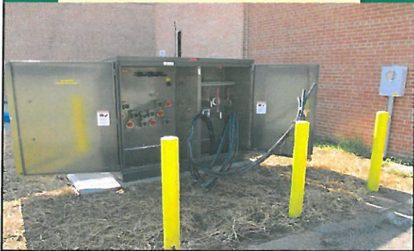
New Electrical Service—North
